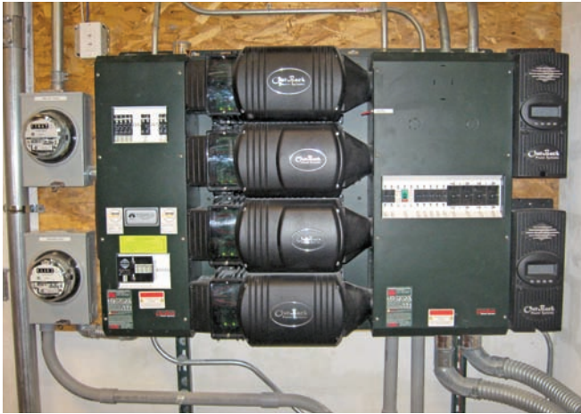
This large home system uses four OutBack charger/inverters in a 120/240 output configuration. The middle two inverters are mainly used to achieve a C/13 charge rate for 2,200 Ah of batteries at 48 V.
